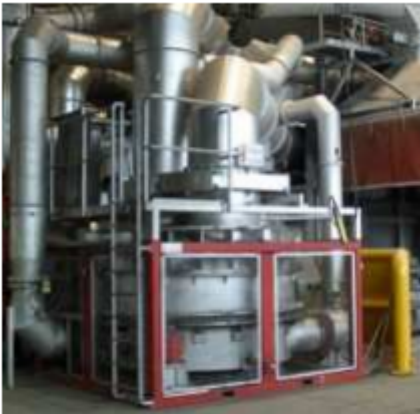
Fig 2 – Rotary regenerator on a Melting Furnace
