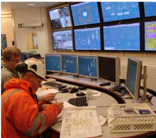
Operators in a processing plant control room
